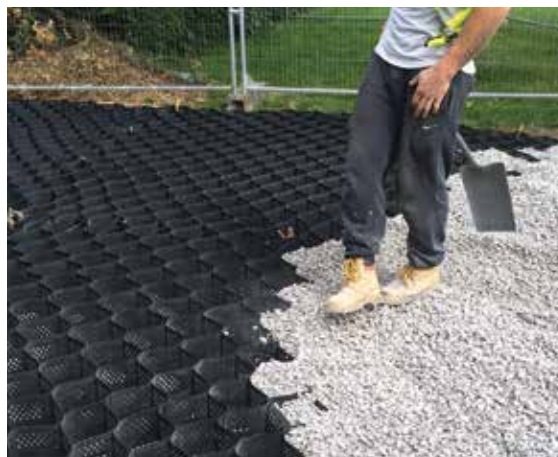
Figure 19.9 Pinning out of cellular confinement system and aggregate infill (courtesy Infra Green Solutions Limited)
