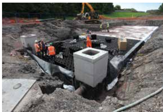
Figure 21.5 Man access chambers located within the structure (courtesy Aco Limited)
